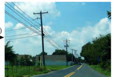
Medium & Low Voltage Distribution Line
