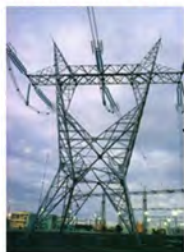
Extra High Voltage Transmission Line
